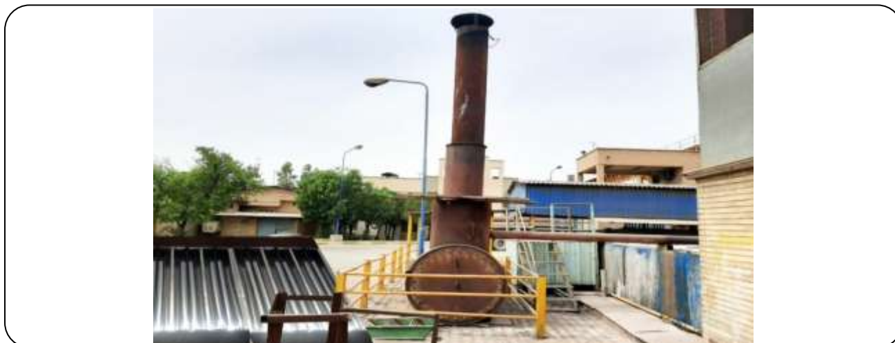
Fig. 1: Solar hot water production system of Dezfoul Industrial Town No. 2.
