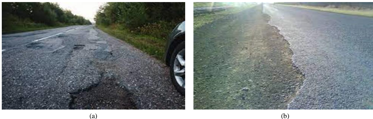
Fig. 1: (a) Raveling of the pavement due to asphalt binder ages (b) Edge cracks in roads due to ingress of the water in underlying layers
