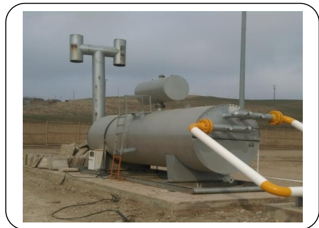
Fig. 2: Indirect heat exchanger (preheater).
