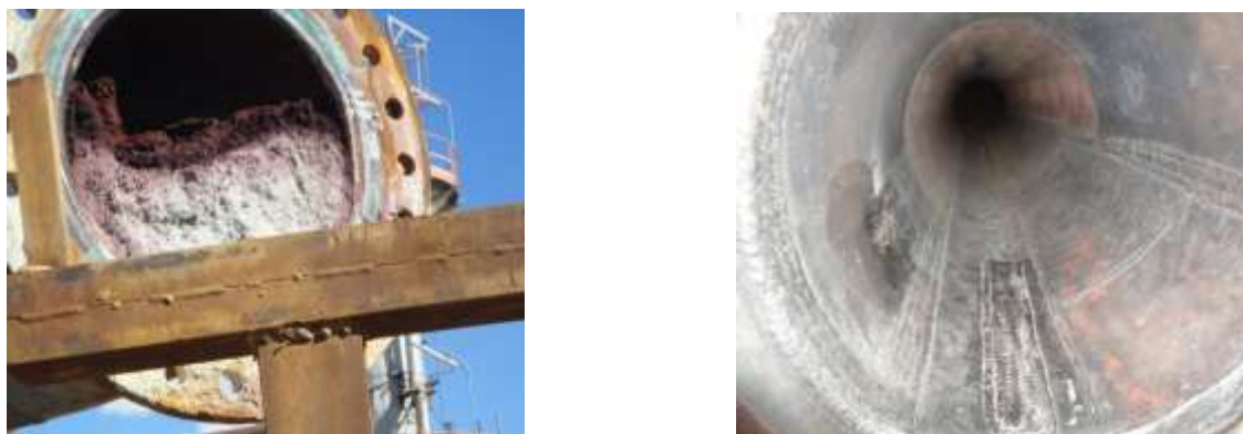
Fig. 5: A) Cross-section of the overhead line with huge amounts of sediments and impurities. B) The cross sectional of the overhead line without deposits after welding.
